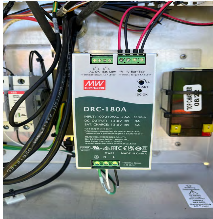
A/C to D/C Transformer
