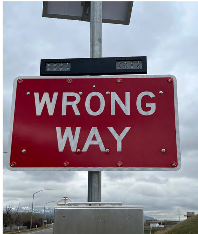
Flashing sign with RRFB
