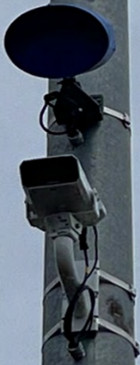
Radar and Intersection Camera
