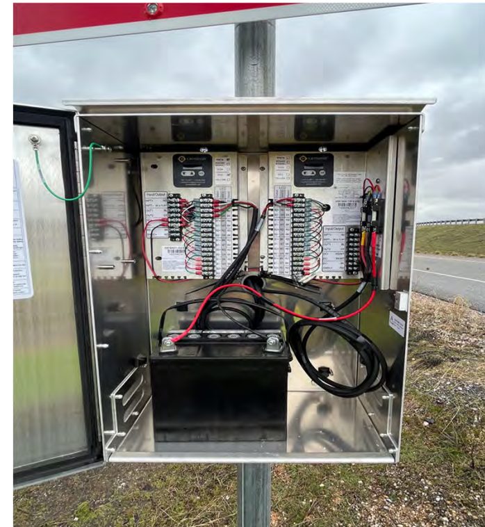
RRFB and LED Solar cabinet
