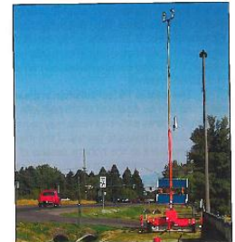
Trailer performing queue detection for traffic management before a campus sports event.
